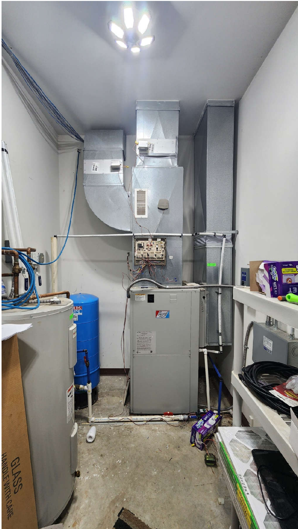
Figure 3 Existing Geothermal System
