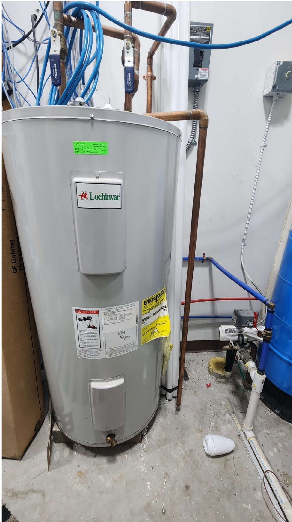
Figure 5 Existing Water Heater
